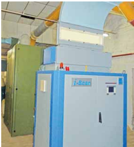
A view of newly installed i- scan machine and unimix.
