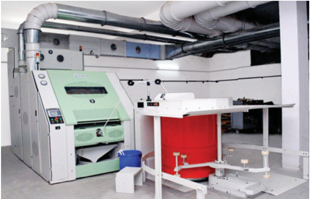
A view of the new LC363 Carding Machine installed at our Mill.
